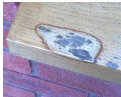
Staining can be sanded out using a detail sander and the coating system reinstated
