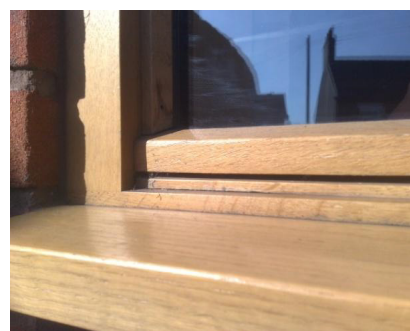
Gaps and exposed end grain should be sealed with Teknoseal products before the coating is reapplied
